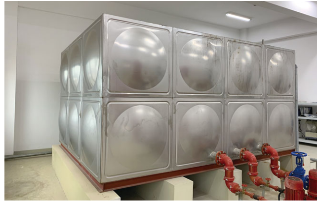
Water Reuse Equipment
